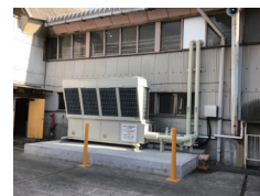
The new chiller
