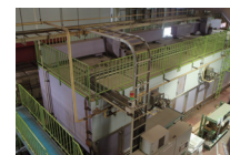
Exterior-clad insulation on the drying furnace door
